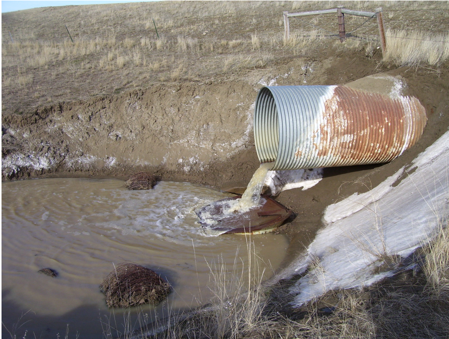
Figure 2 – Scour hole at downstream end of culvert
