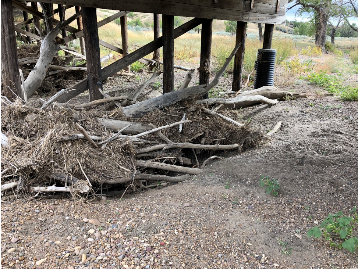
Figure 15 – Debris around bridge pilings
