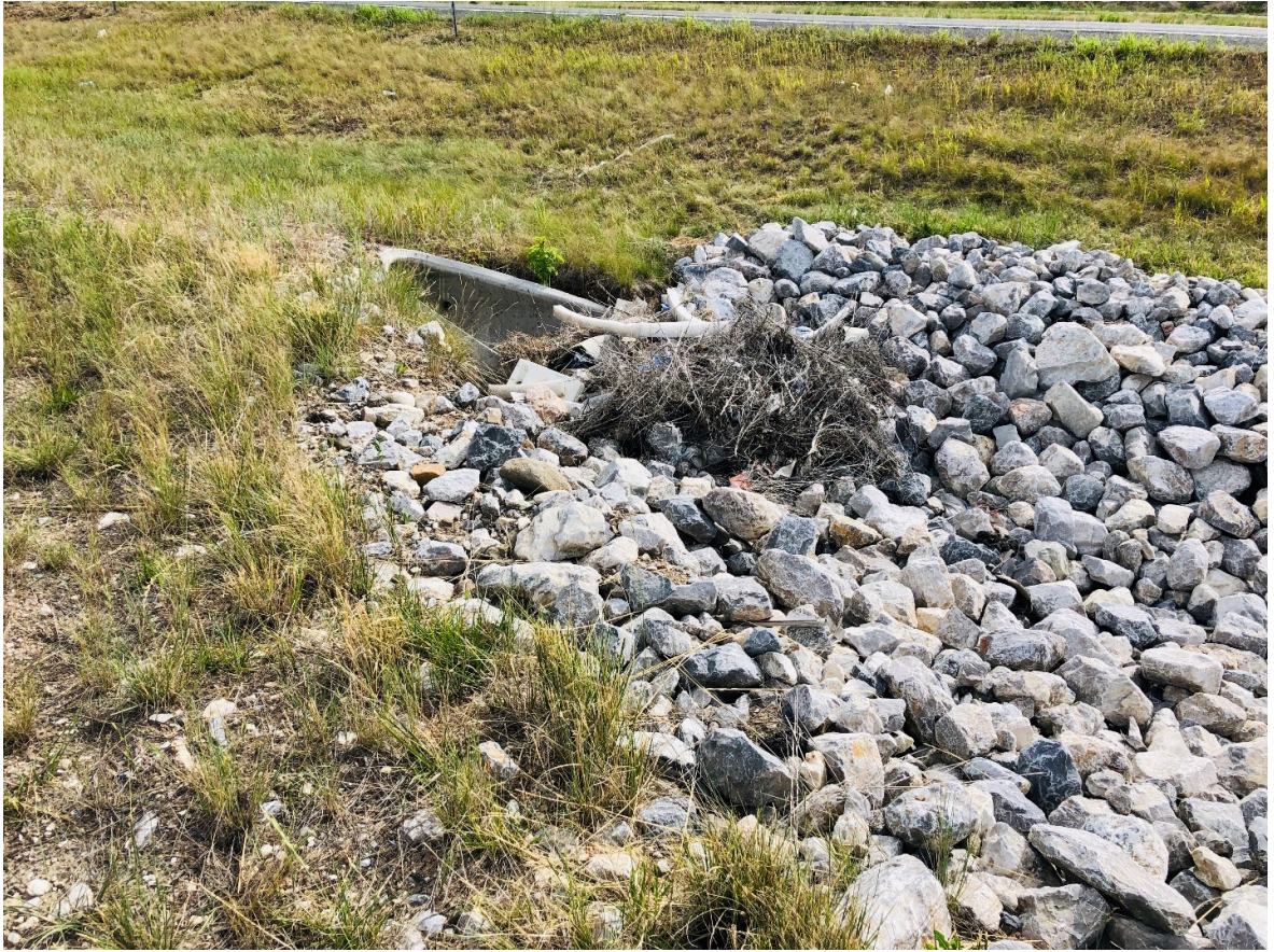
Figure 18 – Pipe outlet with debris accumulation
