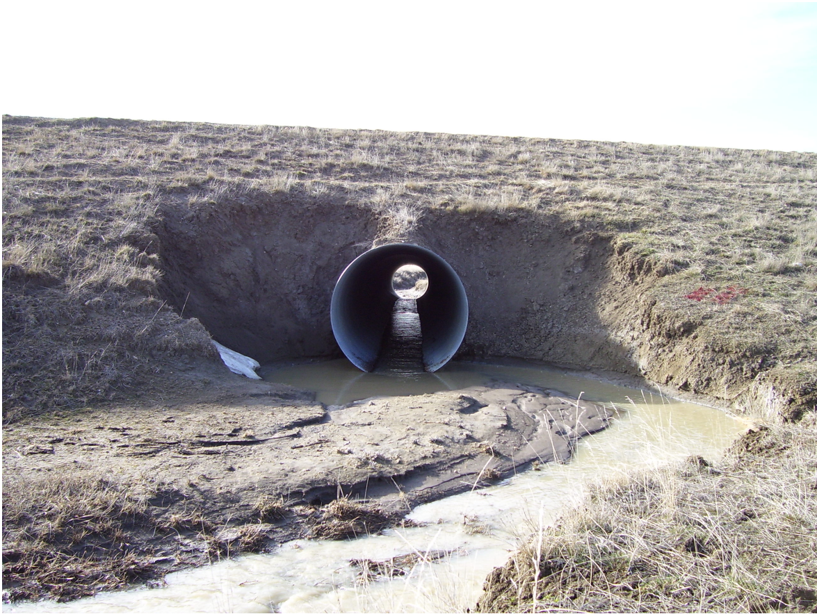
Figure 3 – Erosion at the inlet to a culvert
