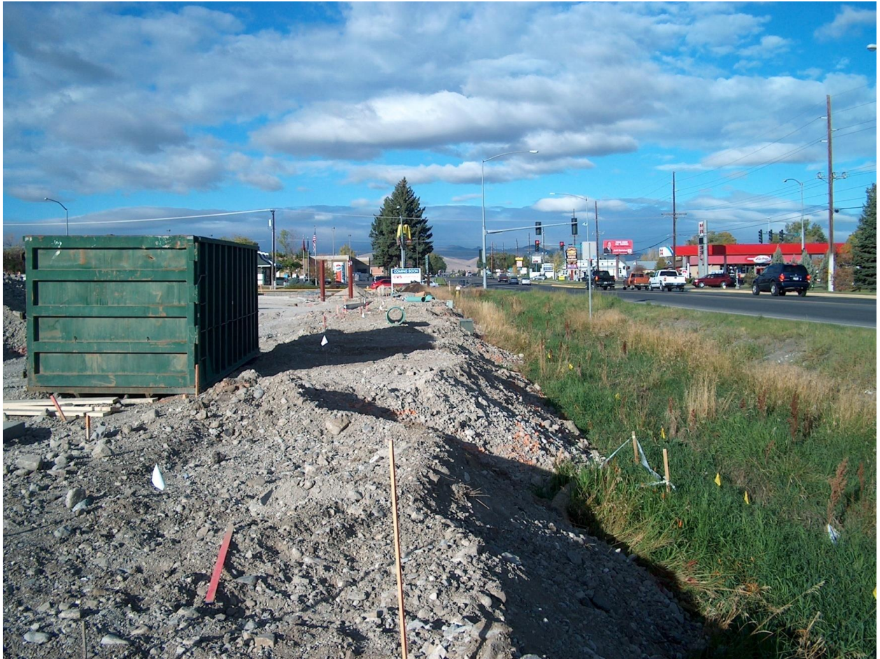
Figure 35 – Construction without BMPs
