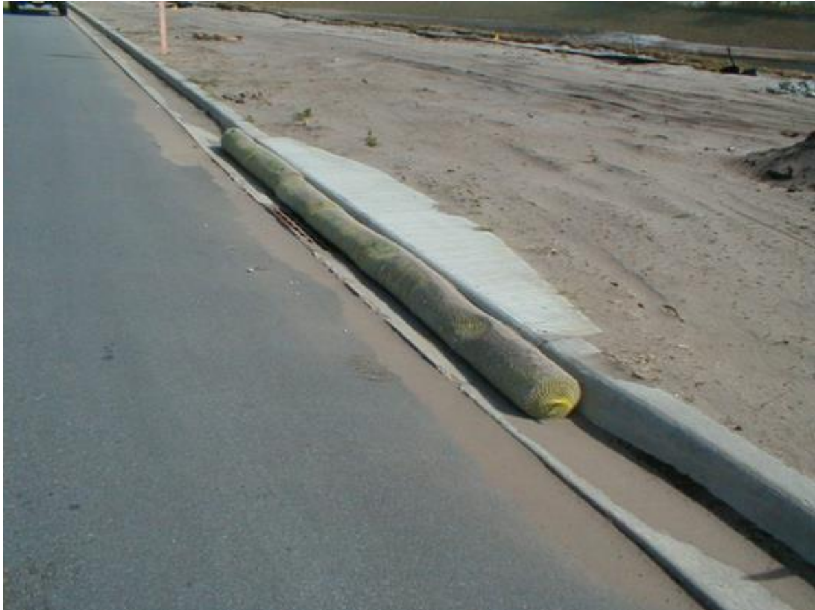
Figure 23 – Straw Log in front of Storm Drain Inlet
