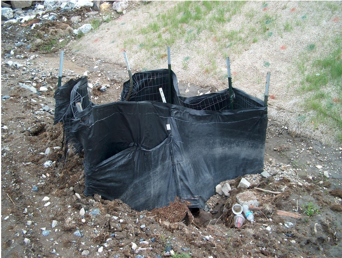
Figure 30 – Silt Fence around an Inlet
