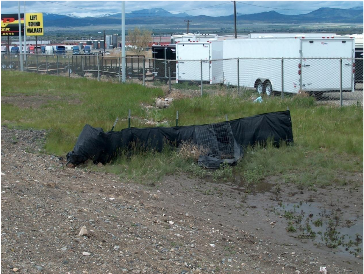
Figure 10 – Silt Fence in Roadside Ditch
