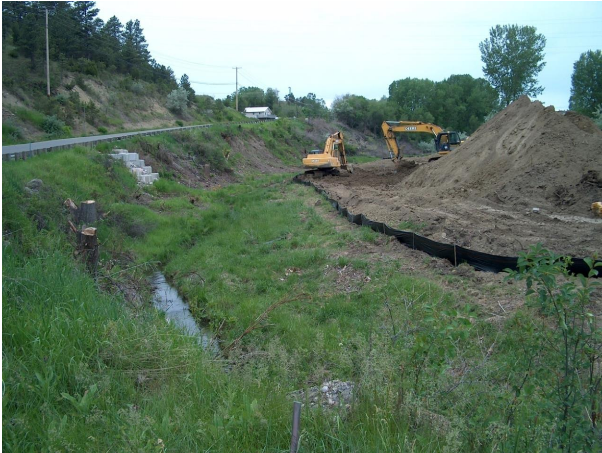
Figure 8 – Silt Fence along a Channel
