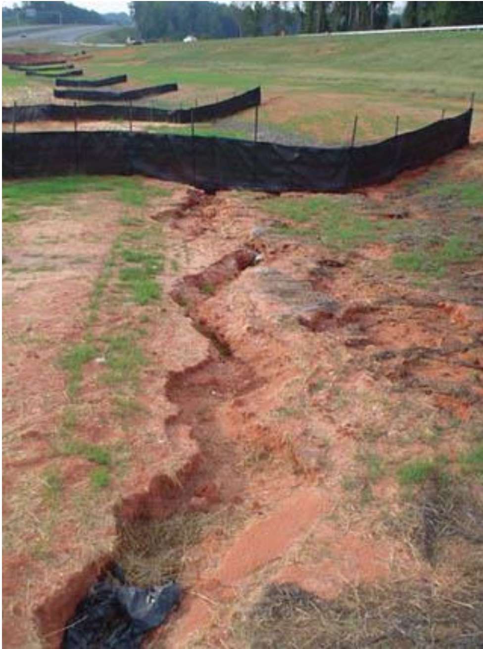
Figure 11 – Silt Fence across a drainage channel
