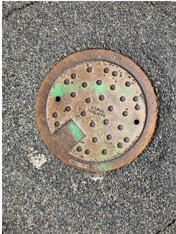
Figure 10 – Manhole Cover with Vent Holes
