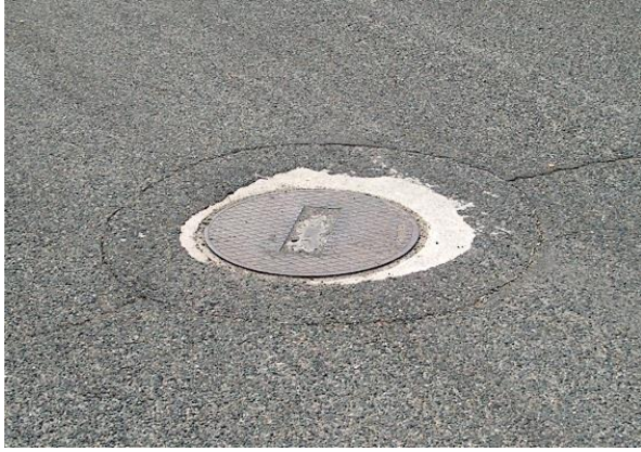
Figure 4 – Typical manhole cover
