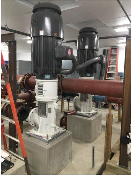
Figure 3 – Vertical Turbine Pump in Service
