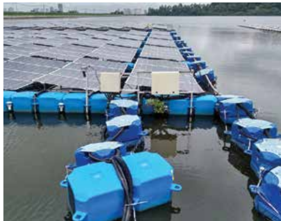
FIGURE 9.6 Vegetation growth due to the spreading of seeds by air, water, or bird droppings
