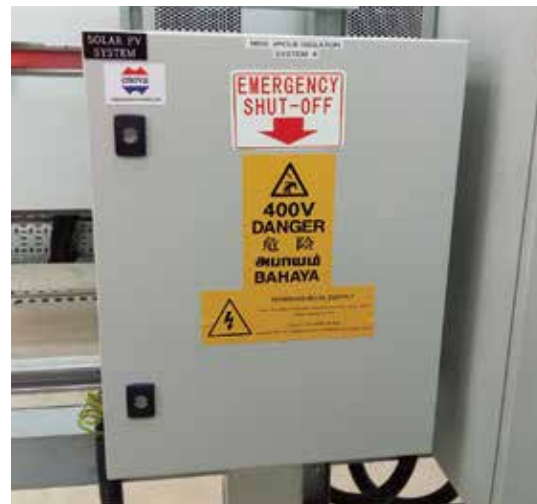
FIGURE 8.11 AC isolator with emergency shutoff
