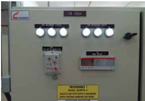
FIGURE 8.8 LED indicating grid supply and FPV supply
