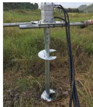
Source: © Ciel & Terre International.
