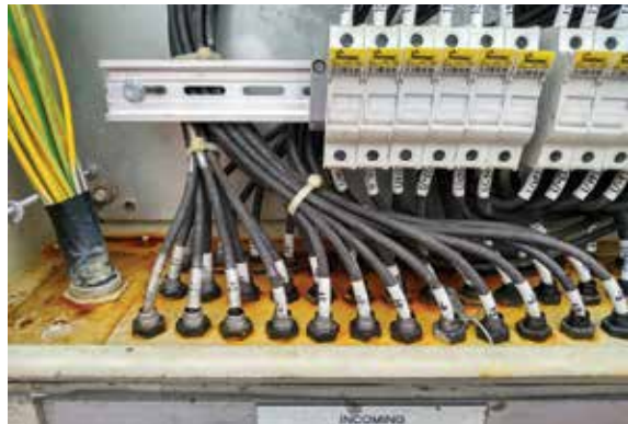
FIGURE 9.19 Water ingress and IP integrity compromised
