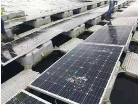
Source: © Lightsource BP Floating Solar Array, London.
