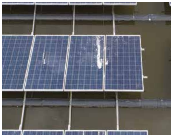
FIGURE 9.5 Severe bird droppings at a testbed in Tengeh Reservoir, Singapore
