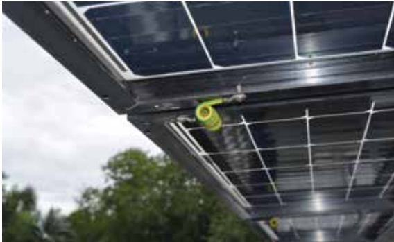
FIGURE 4.17 Equipotential bonding, Singapore Tengah Reservoir testbed
