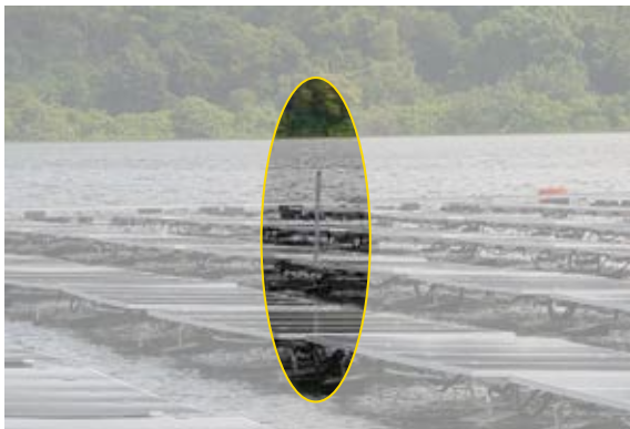
FIGURE 4.15 Air terminal rods installed on an FPV island, Singapore Tengah Reservoir testbed
