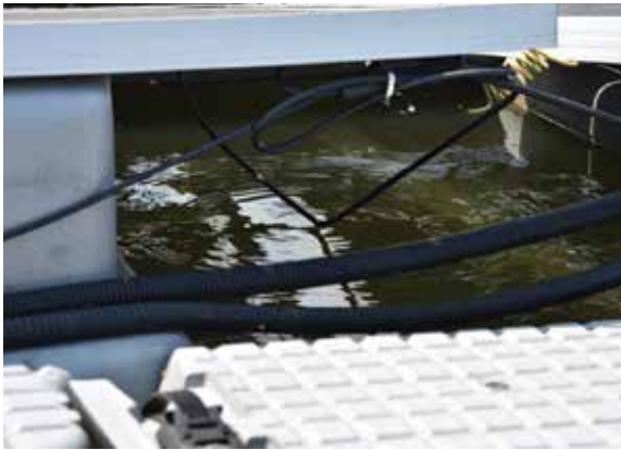
FIGURE 7.6 Examples of cables in contact with water
