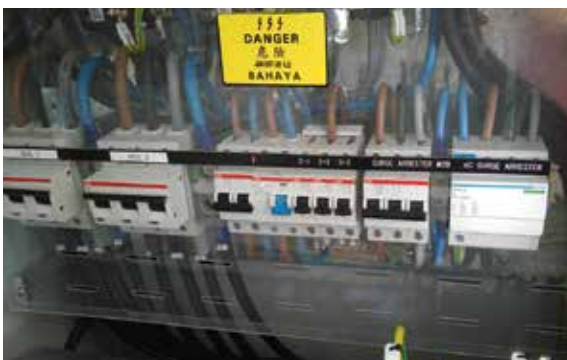
FIGURE 8.9 AC subboard with surge protection device
