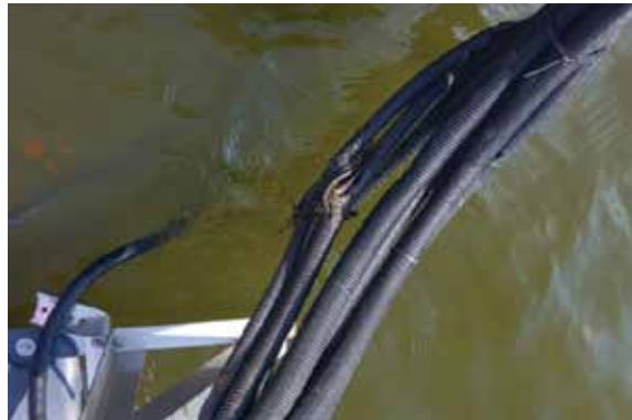
FIGURE 9.18 Conduit and cable sheath wear out
