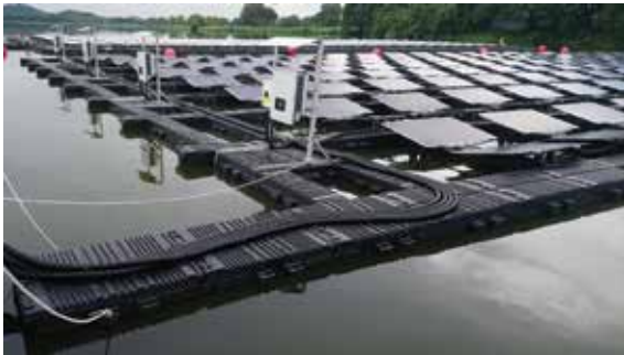
FIGURE 4.2 Layout of FPV systems with string inverter placed on floats, Singapore Tengah Reservoir testbed
